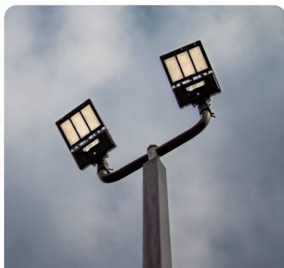
FL05 Area Lights
